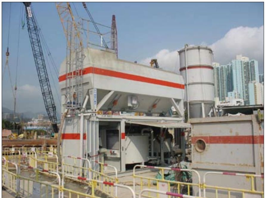
Another motor pump MP7 in the construction site of the underground station of Sham Shui Po District, the dense underground network in Hong Kong
