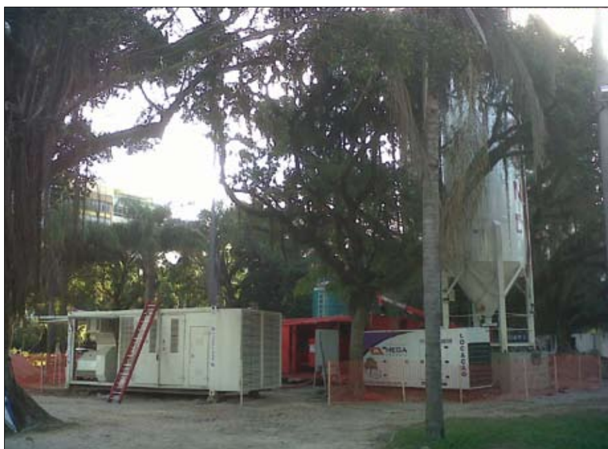
The construction works of new underground stations in Rio de Janeiro, here that of Nossa Senhora da Paz. Metax participated with its equipment at different construction sites, in particular by providing different types of motor pump MP7
